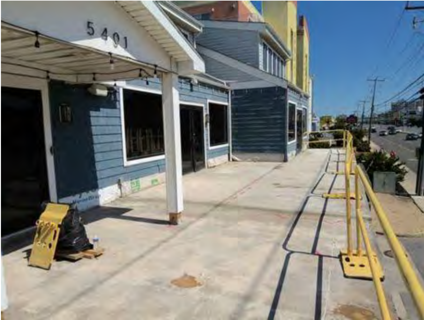
Looking from the stairs to the front entrance, door #2 and door #3 entrances to the premises.
